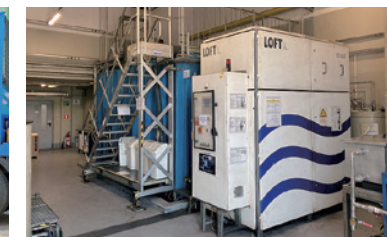
Liquid waste evaporation system
